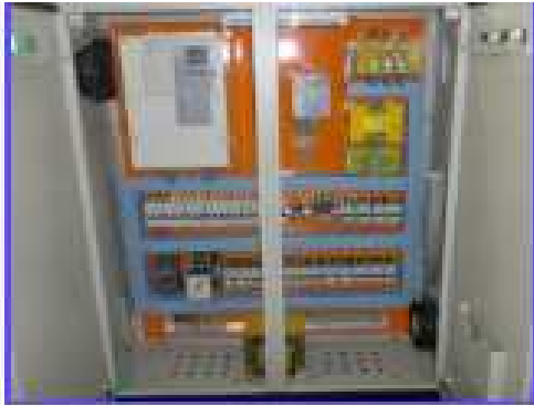
Electrical Panel With VVVF Drive
