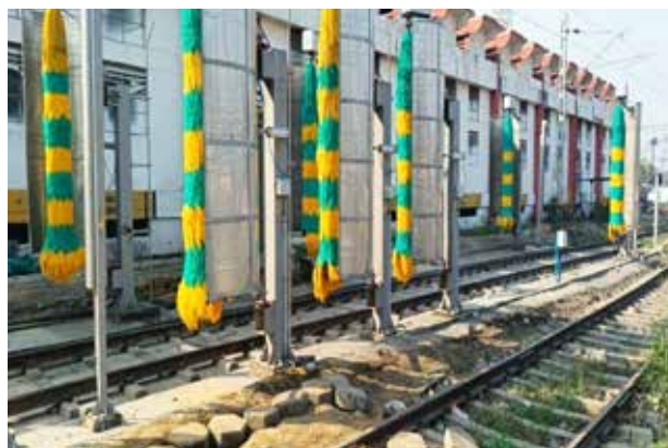
ACWP at JUC DEMU Car Shed
