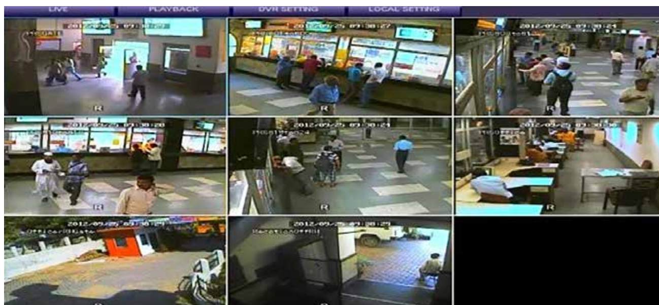
(CCTV at Lucknow station)
